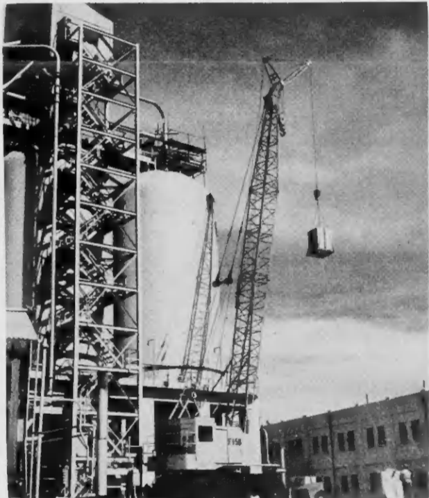
WHEN THE PCAR catalyst elevator failed recently, a crane was substituted to lift catalyst to hoppers. ORA CU e lift di catalyst a faya recientemente, un grua a worde substituí pa hiza catalyst pa hoppers.
